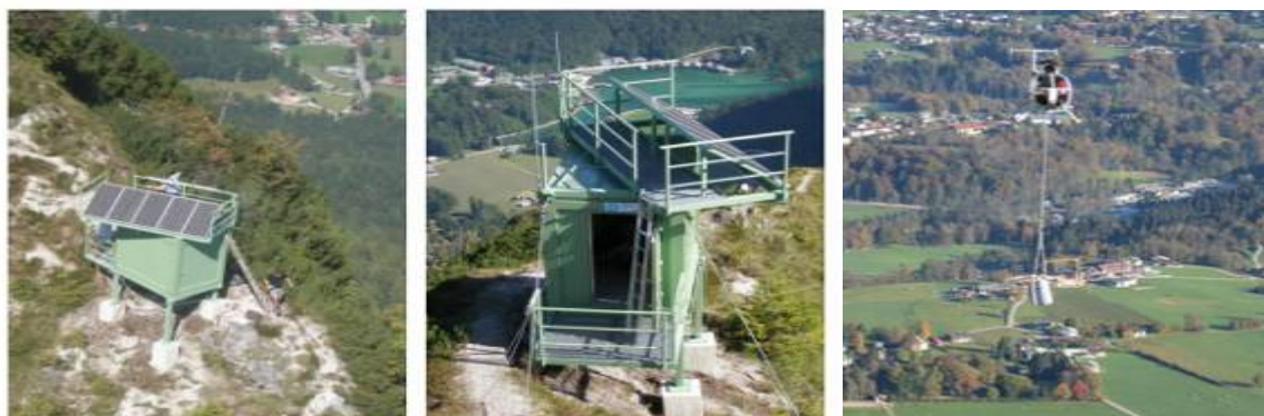
Fig. 4 Transmit Station at the Gruenstein mountain and Helicopter transport of GTS rack
