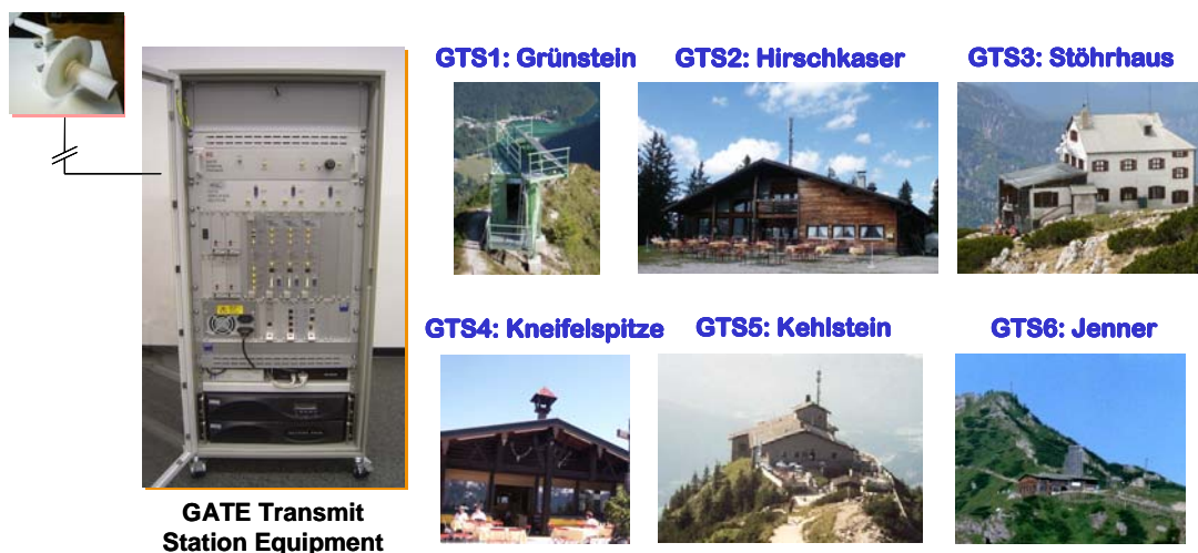
Fig. 2 GATE Transmitter Locations and Transmitter Rack GATE Infrastructure Overview
